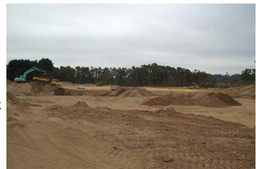
Construction of a spillway to protect the Avon River & surrounding properties from flood damage.
